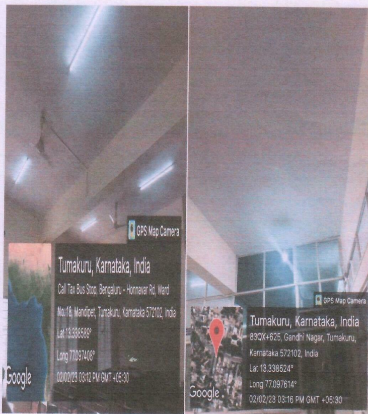
Photo of LED Bulb in Staff Room
