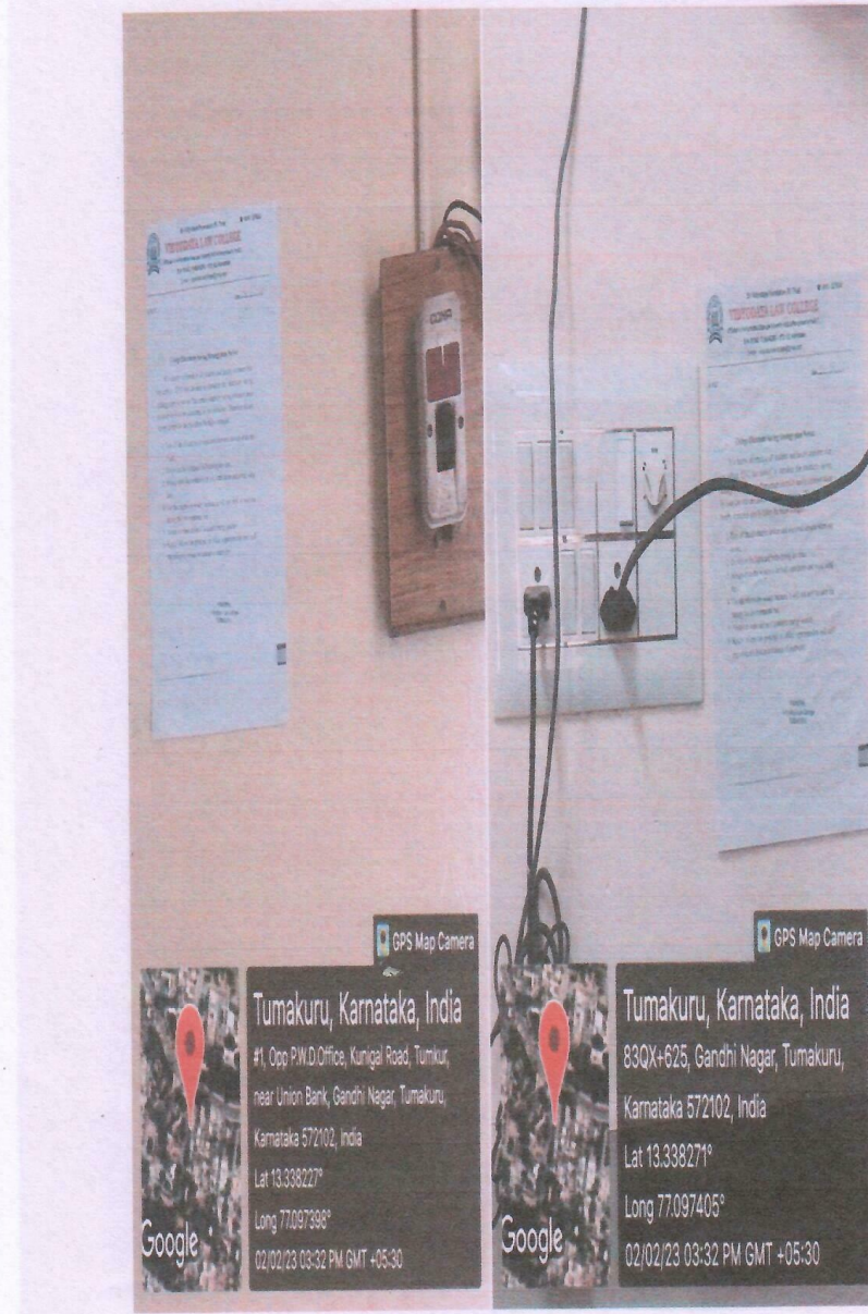
Photo of the Energy Saving Notices displayed near Switch Boards
